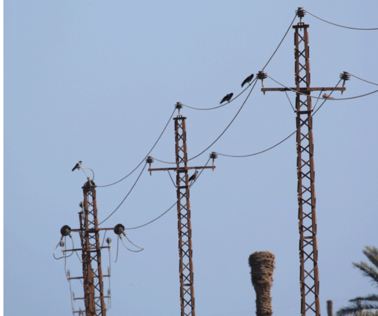
Figure 6. This is the most widespread low voltage distribution OHTL setup in Egypt, with short upright insulators. This line was photographed in Fayoum
