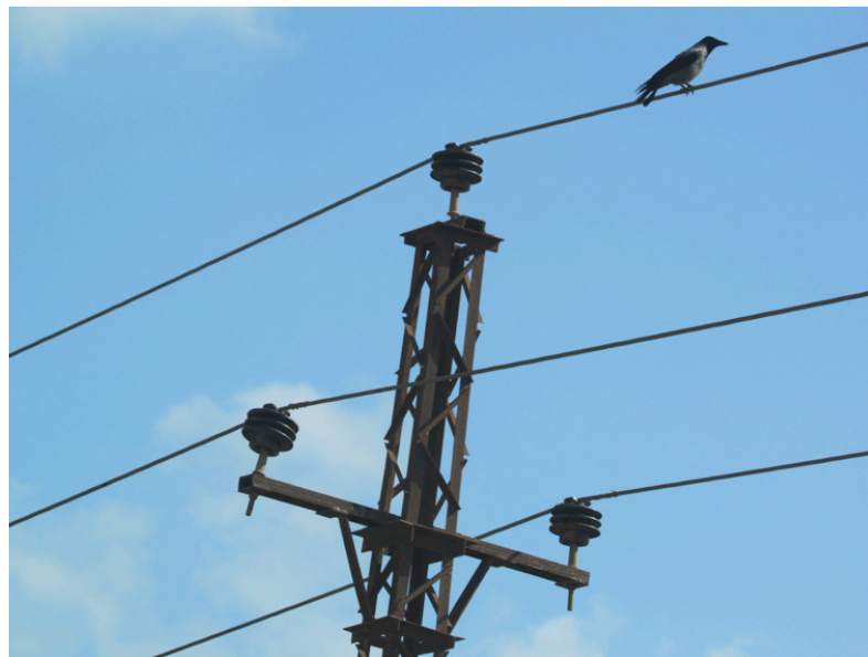
Figure 7. The typical distribution power poles throughout Egypt, have metal lattice structure and a cross bar with very short insulators that are about 40 cm high. These
