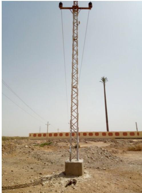
Figure 8. Steppe Buzzard electrocuted when landing on a 66 kv pylon with short upwards insulators at Ain Sukhna. There are at least 17, 500 km of such power lines in Egypt, making it the most common component of the power transfer network in the country.
